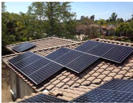
7.5KW Grid Power Station
