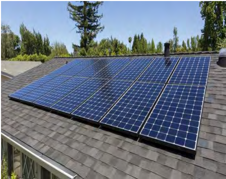
5KW Grid Power Station
