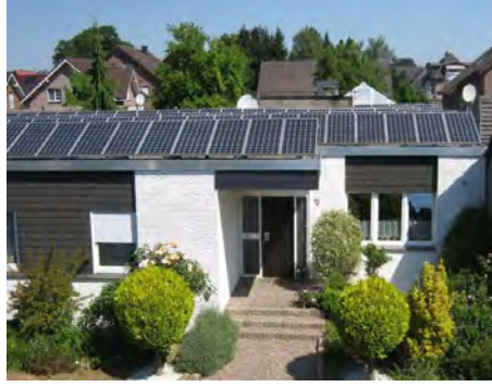
15KW Grid Power Station
