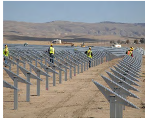
1.6MW Grid Power Station
