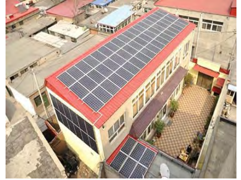
20KW Grid Power Station
