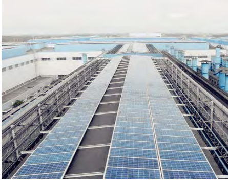
200KW Grid Power Station
