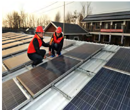
220KW Grid Power Station
